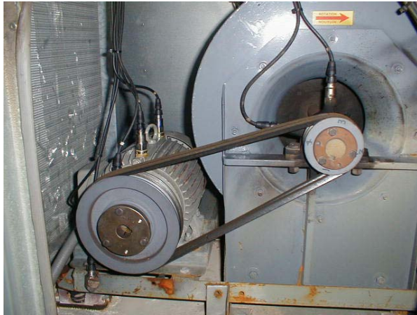
Permanent Accelerometers Placed on Motor and Fan Bearings
